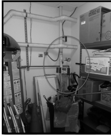
Figure 21 Sprinkler Riser is Blocked in a Storeroom
